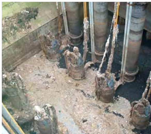
Pump station with accumulation of floating debris.
